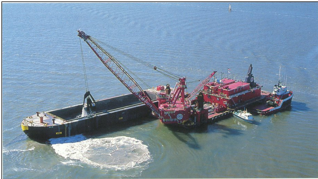
Figure 17: The largest clamshell grab used in dredging, the Chicago, in full operation.
